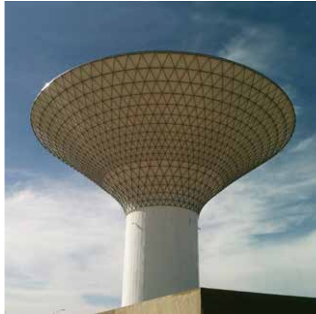
Water tower Leon, Mexico: Sikaplan® WT-4220.
