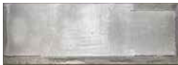
Mortar with good crack behavior.
